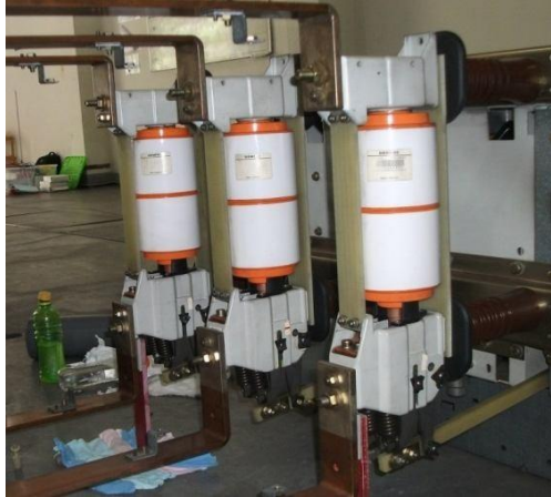
Figure 2.3 20 KV Cubicle Power Circuit Breaker
