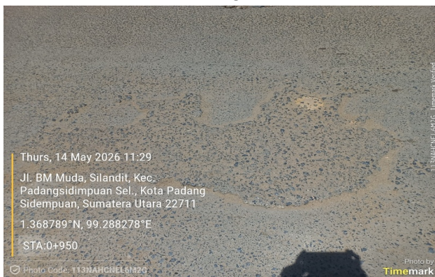
Patch on Segment 20
