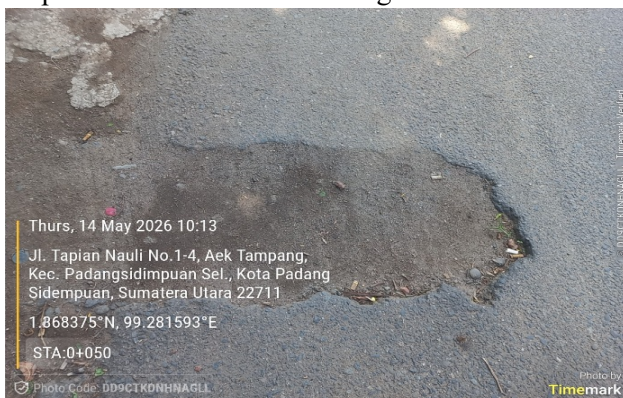
Hole in Segment 2
