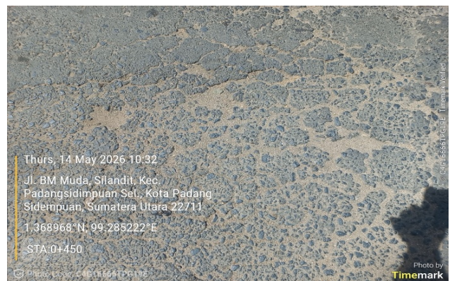
Crocodile skin crack on Segment 10
