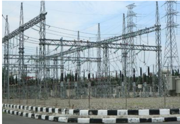
Figure 27 Substation Sei Mangkei Parent Source: Author's Documentation
