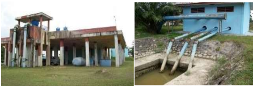
Figure 4.3 Condition of Water Treatment Plant Infrastructure and Pipe Network (Source: Documentation of the PUTR Service of Tanjungbalai City, 2025)
