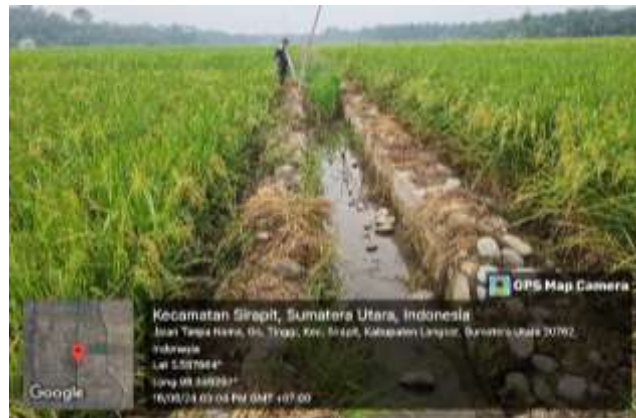
Figure 4.1. Structural Damage to Channels
